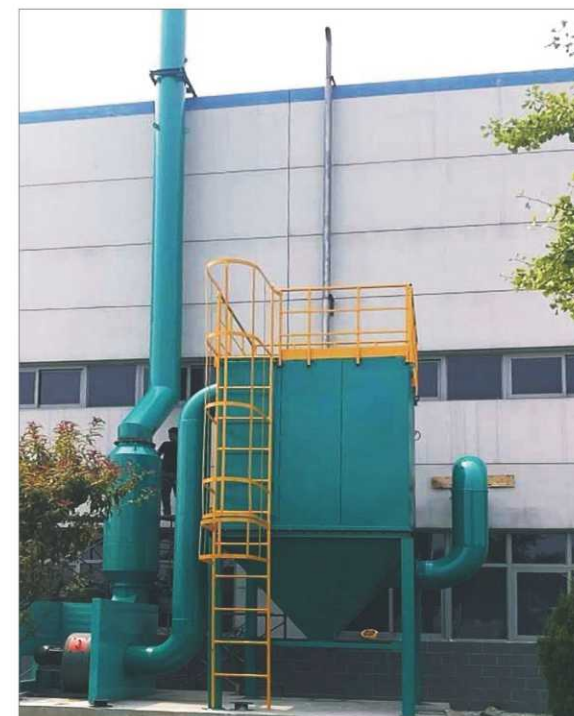
Pulse Cloth bag Dust Removal Equipment and Noise Reduction Facilities
