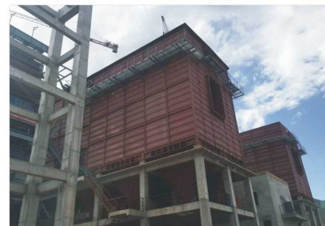
Production and Installation Site of 220 Ton Circulating Fluidized Bed Boiler Dust Collector
