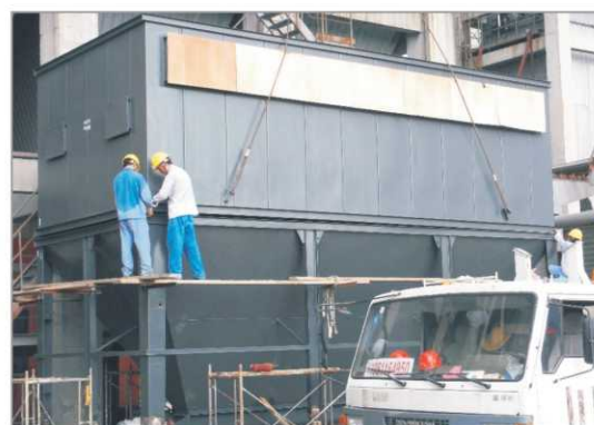
Boiler Supporting Ceramic Multi-tube Cyclone Dust Collector
