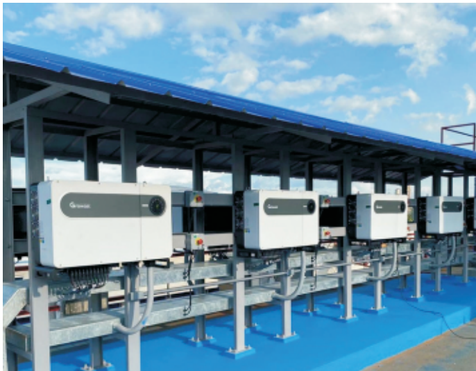
CASE STUDY: Philippines with 1.2MW solar installation.
